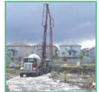
Stabilized construction exit.
